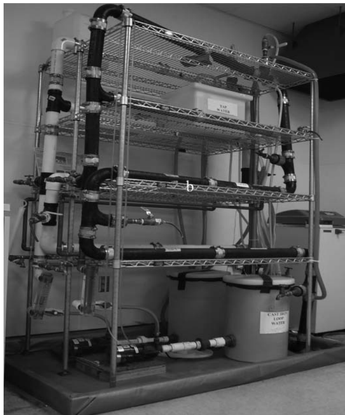
Fig. 1. Cast-iron and PVC model distribution systems.
